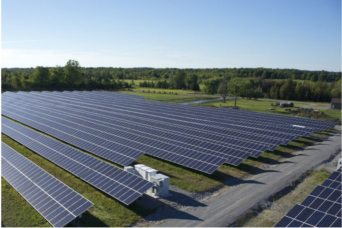
Plate 4.2 Typical Fixed Panels (with Inverters)
