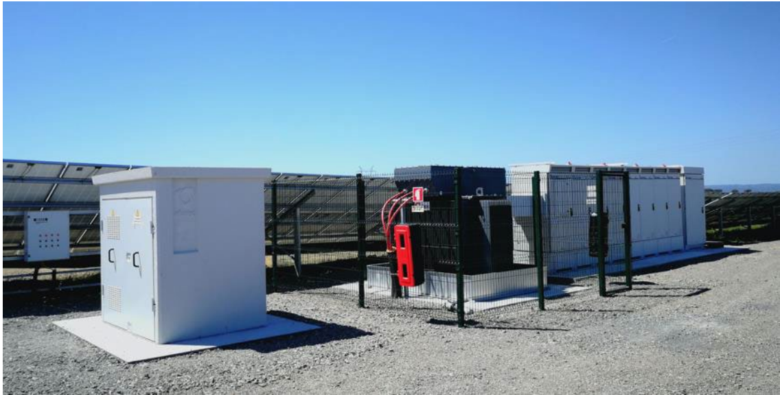
Plate 4.6 Conversion Unit (independent equipment)
