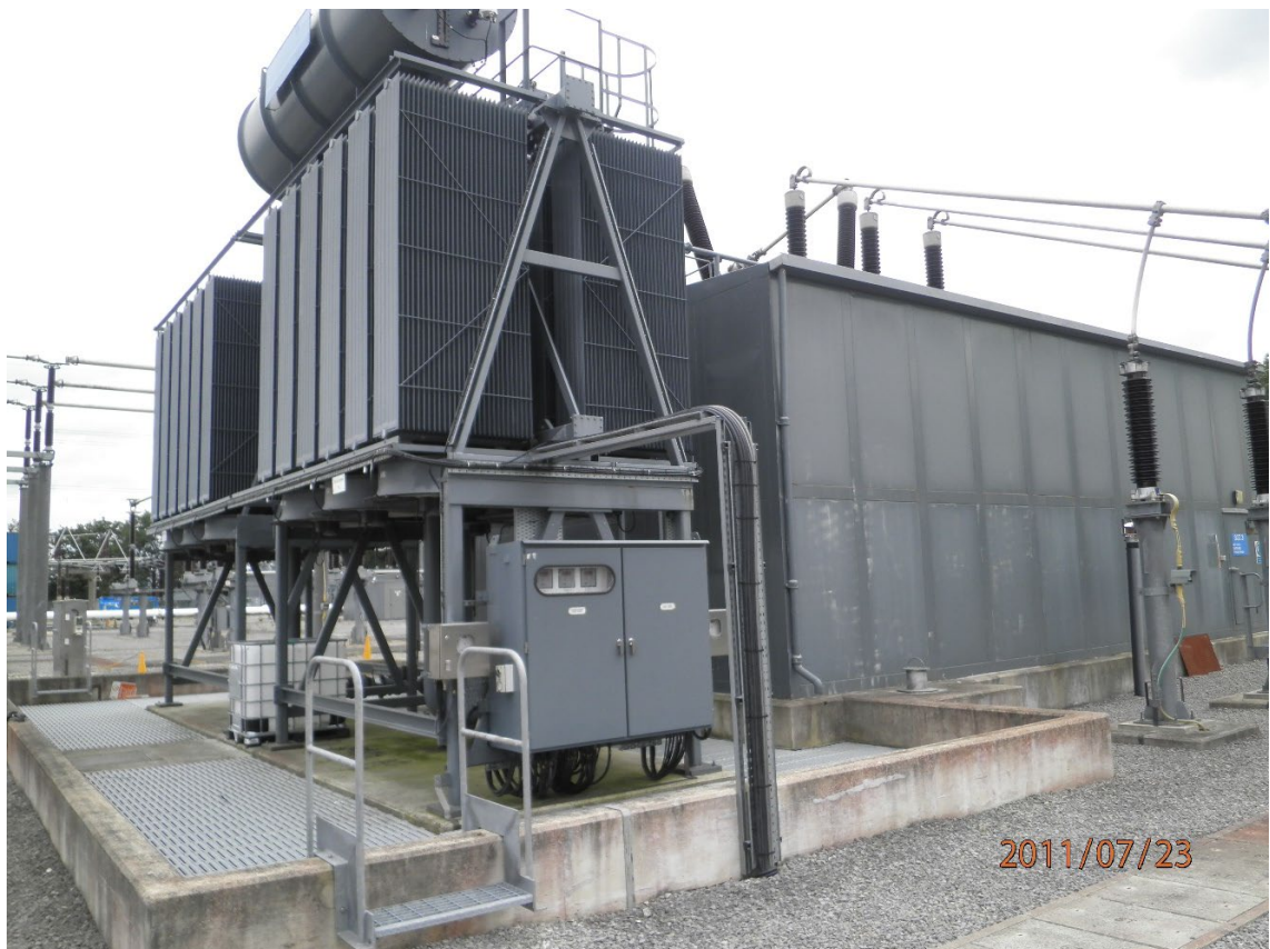
Plate 4.9 Typical (large 400kV) power transformer
