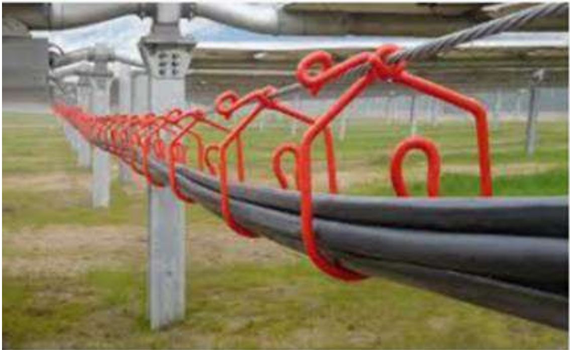
Plate 4.7 Suspended Cabling System
